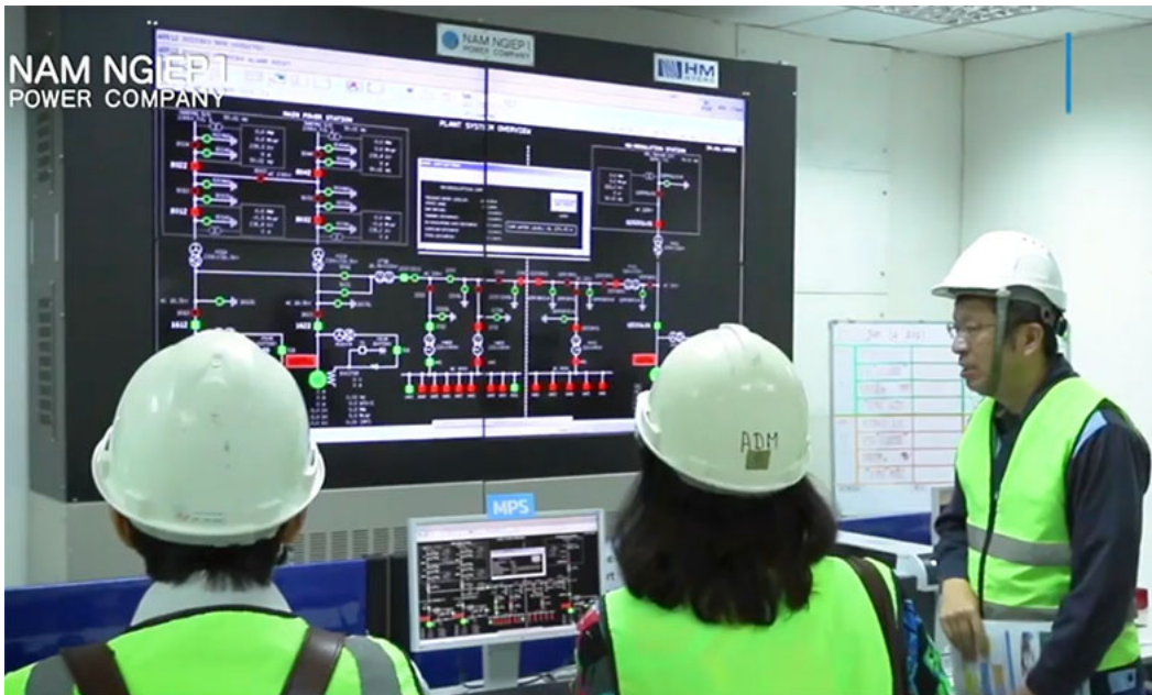
Nam Ngiep 1 powerhouse interior image below:
